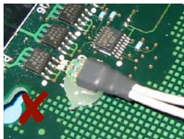
Figure 15 Incorrect Securing Method Because Glue is Placed on the Probe Head Tip
